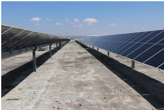
2.4MW Radhanpur solar Plant
